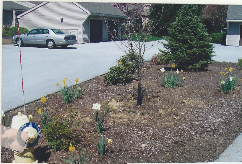
Backflow valves on east end of Fire Hydrant Island + three other locations. Total 6 + 1 Retrofit done 2006 and 2007
